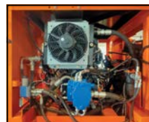
Main Hydraulic Pump
