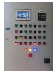
The Control Panel, containing an integral computer
